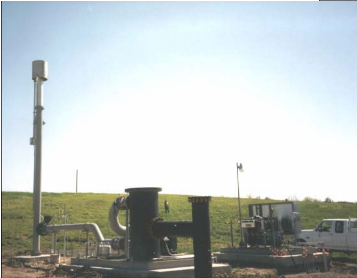
SEMI ENCLOSED LANDFILL FLARE STATION
