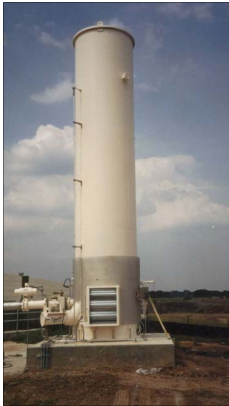
ENCLOSED GROUND FLARE
